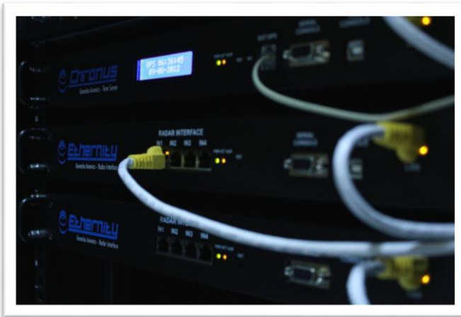
Ethernity Radar Data Interface (Rackmount)
